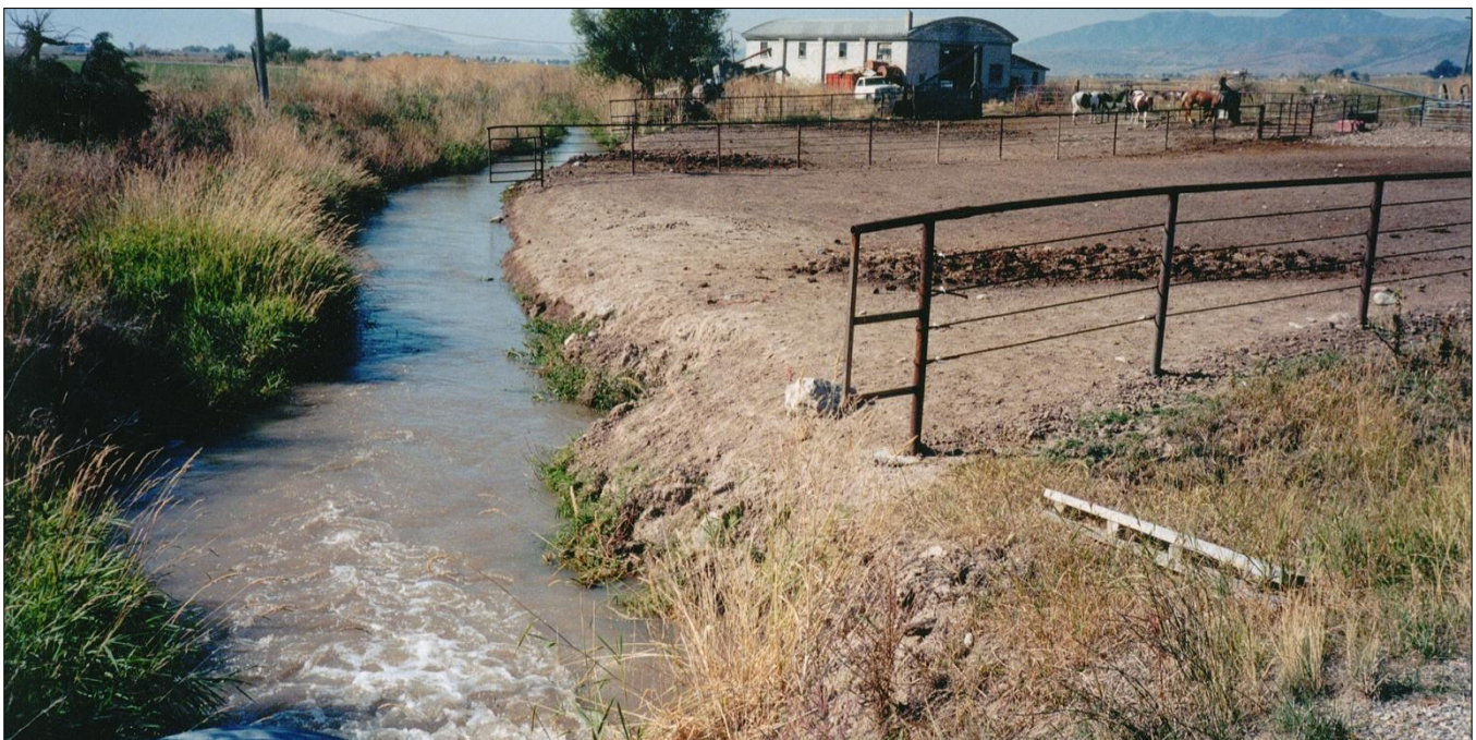
An example of stream bank degradation (Richard Toth)
