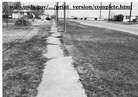
Infrastructure or housing that is built on unstable soils can have detrimental effects, such as this dislocated sidewalk.
